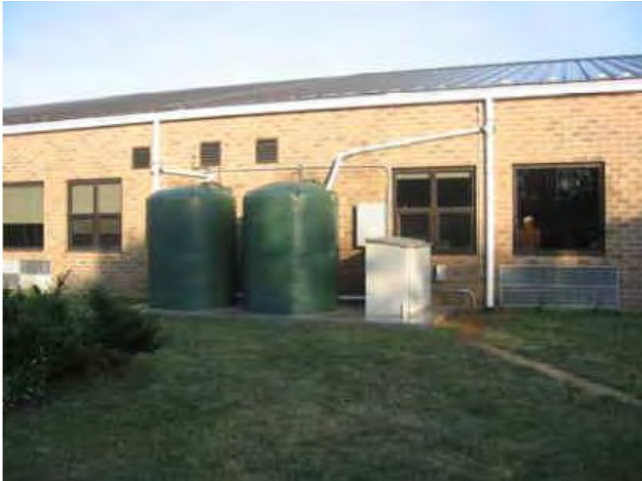
Samuel Mickle School Rainwater Harvesting System
